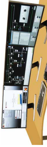
PST2250-15 SCADA System
