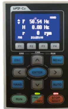
AC Drive Control Panel
